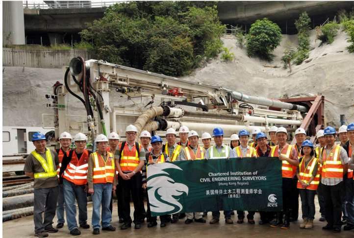
Members and guests were visiting the operations of tunnel boring machines at the tunnel entrance
